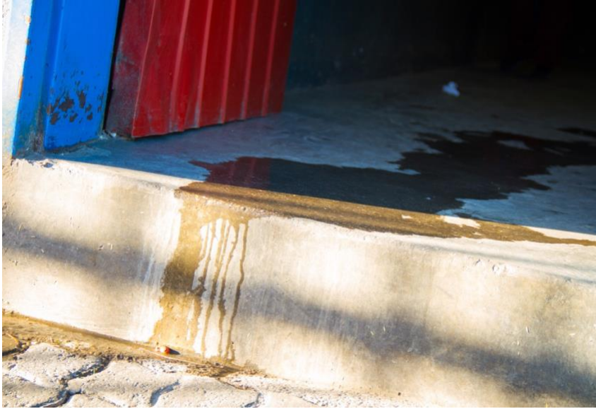
Fig 3. Leakages and running water from restrooms at the Tutungeni Open Market in Okuryangave
